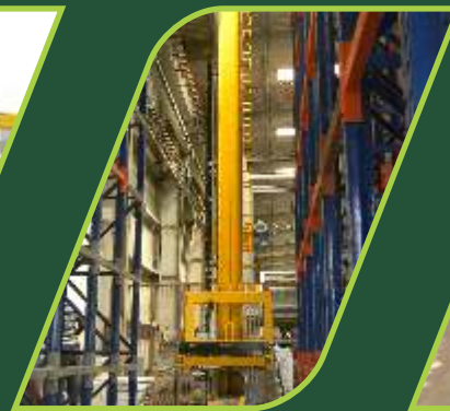
AUTOMATIC STORAGE & RETRIVAL SYSTEM
